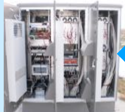
39x NL LOFAR Cabinet 14x International ILT-container
